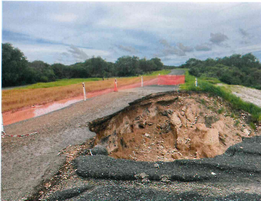
Elim Road Embankment Failure
